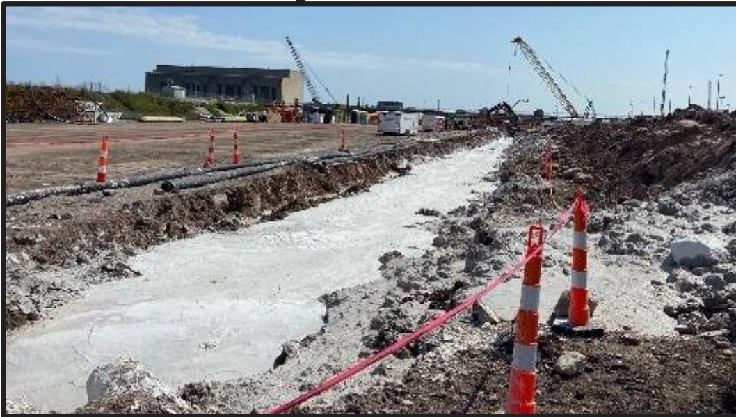
Placement of the Soil Cement – Cement Bentonite (SCCB) wall north of the Sabin Lock to prevent seepage through soil into the dewatered excavation area
