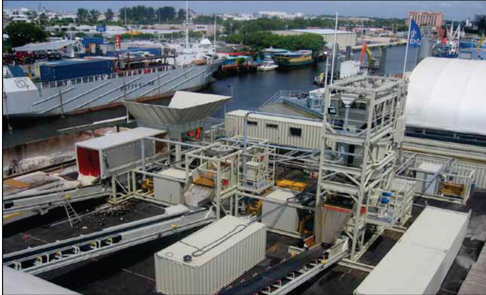
Figure D-3. Photograph of Boskalis-Dolman vibrating screens, hydrocyclones, and sediment processing system, Miami River, Florida (courtesy Bastiaan Lammers, Boskalis Dolman).
