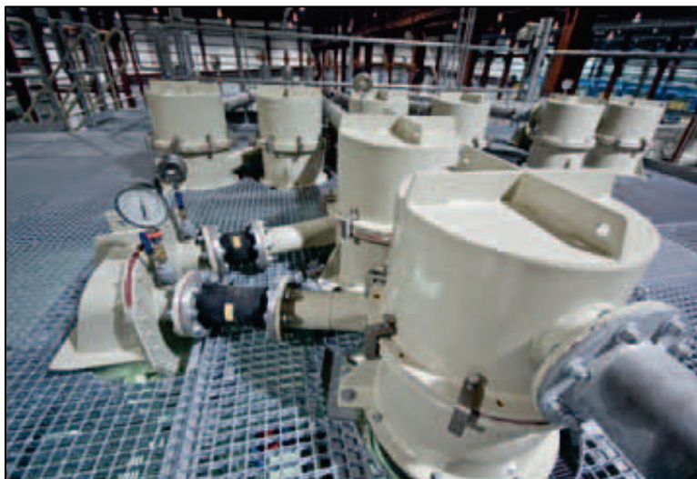
Figure D-7. Hydrocyclones for sand separation.
