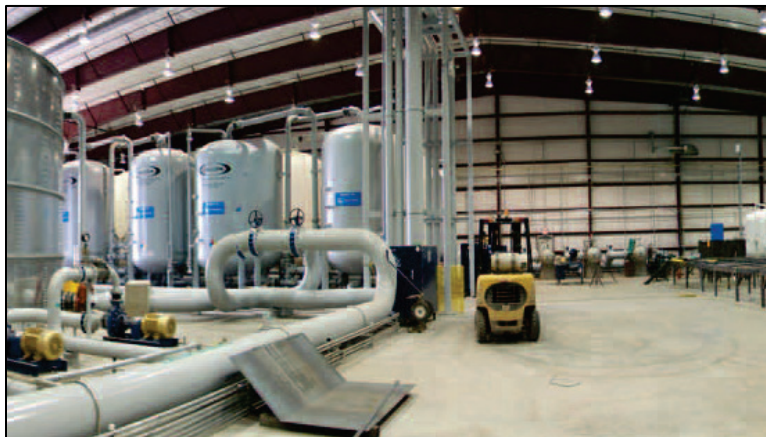
Figure D-9. Water treatment plant, 9000 GPM capacity, sand, bag, and carbon filtration processes.
