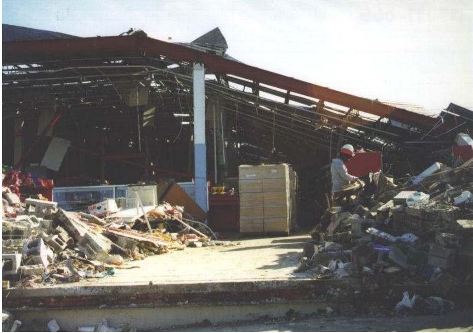
WHB: DOD 7: Total destruction of a large section of building
