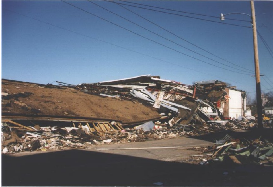
LIRB: DOD 4: Long span roof structure collapses downward
