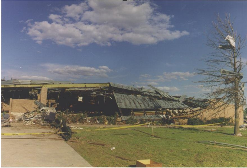
ES: DOD 9: Collapse of load-bearing walls
