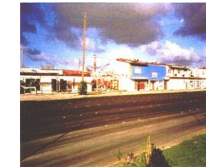
Weakened wood and tin roofs can fail
