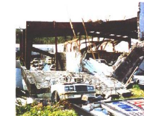
Poorly reinforced hollow-block walls can topple
