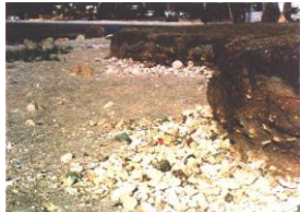
Coastal erosion undermining inland rocks
