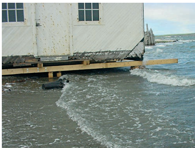
July, 2003 - the NW&TCo Store after the shed addition was removed and the building raised (Credit: Government of Yukon Territory)
