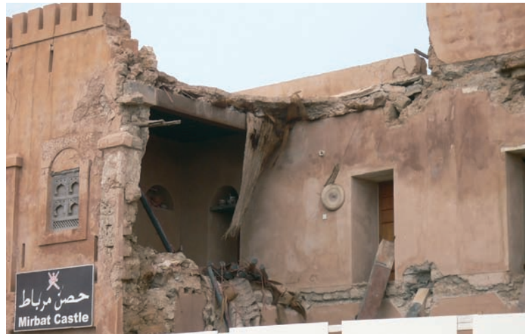
Mirbat, castle with collapsed walls and roof, 2007 (Photo: M.Pz.)
