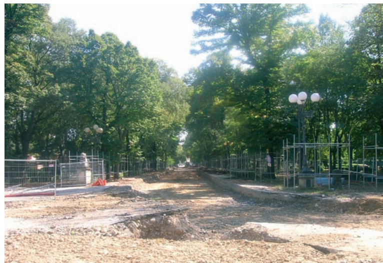
The central alley of elms dug up for the instalment of train rails
