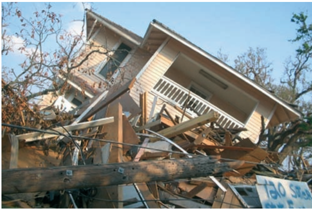
Destroyed house in Biloxi
