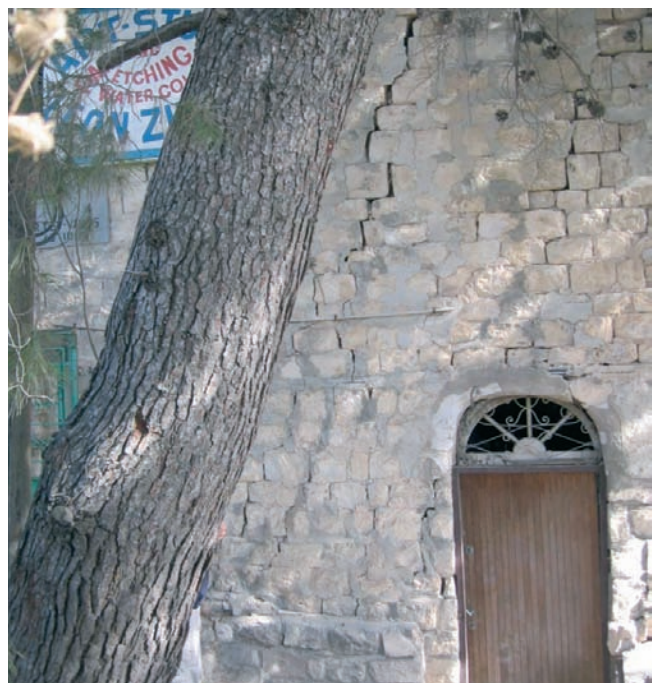
Old Zefat, cracks on an old building in the Maayan area
