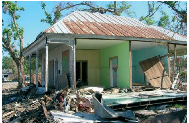
Last house on Pearl Street, Biloxi
