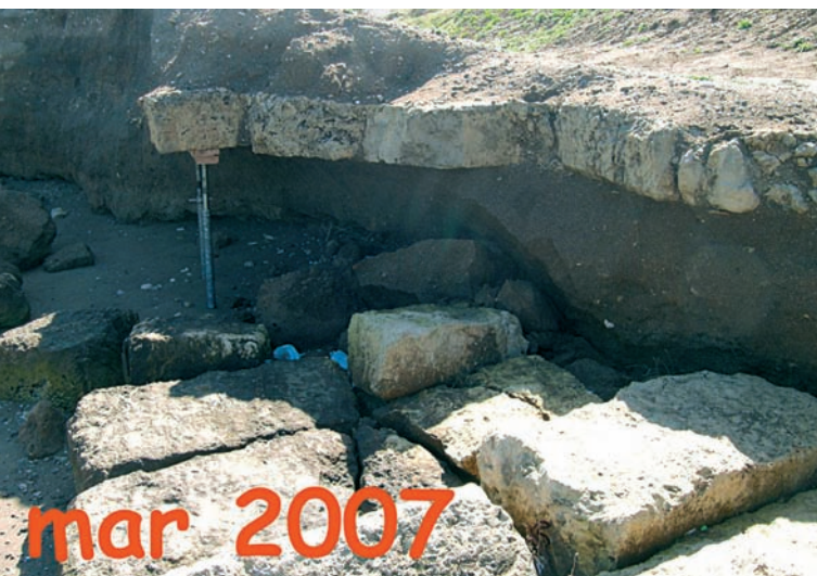
One of the two points supported at the beginning of March 2006 by the Direction for the Restoration of Ancient Monuments.
