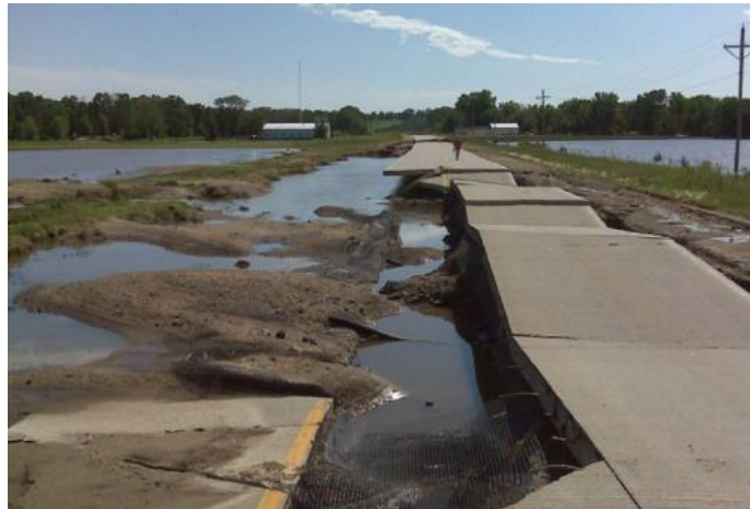
FIGURE 16: IA-1 FLOOD DAMAGE NEAR MOUNT VERNON, IOWA.
