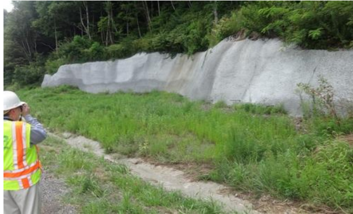
FIGURE 28: COMPLETED TOE WALL AT THE BASE OF THE SLIDING MASS AT I-77, MP 1.8 , VA I-77.
