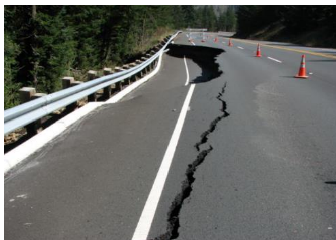
FIGURE 15: PAVEMENT FAILURE AFTER FLOODING ON US-101 SOUTH OF GOLD BEACH, OREGON.
