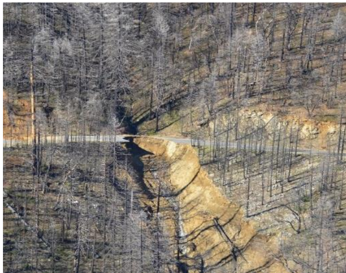
FIGURE 22: ROADWAY BREACHING AFTER FLOOD EVENT IN A POST-WILDFIRE WATERSHED, CALIFORNIA.
