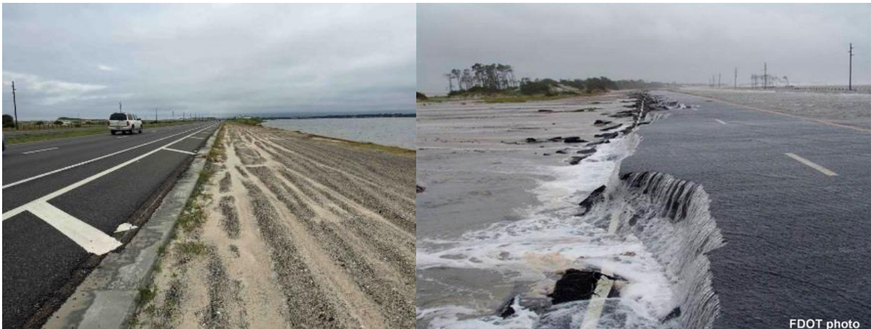
FIGURE 13: COASTAL CLIMATE CHANGE ADAPTATION MEASURES WILL BE SIMILAR TO COASTAL ENGINEERING STRATEGIES FOR IMPROVING RESILIENCE TO TODAY'S EXTREME WEATHER EVENTS.
