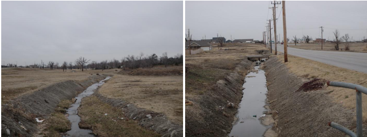
Figure 10: Photos of the existing Joplin Creek through Campbell Parkway (left) and as a channelized ditch near South Highview Avenue (right).
