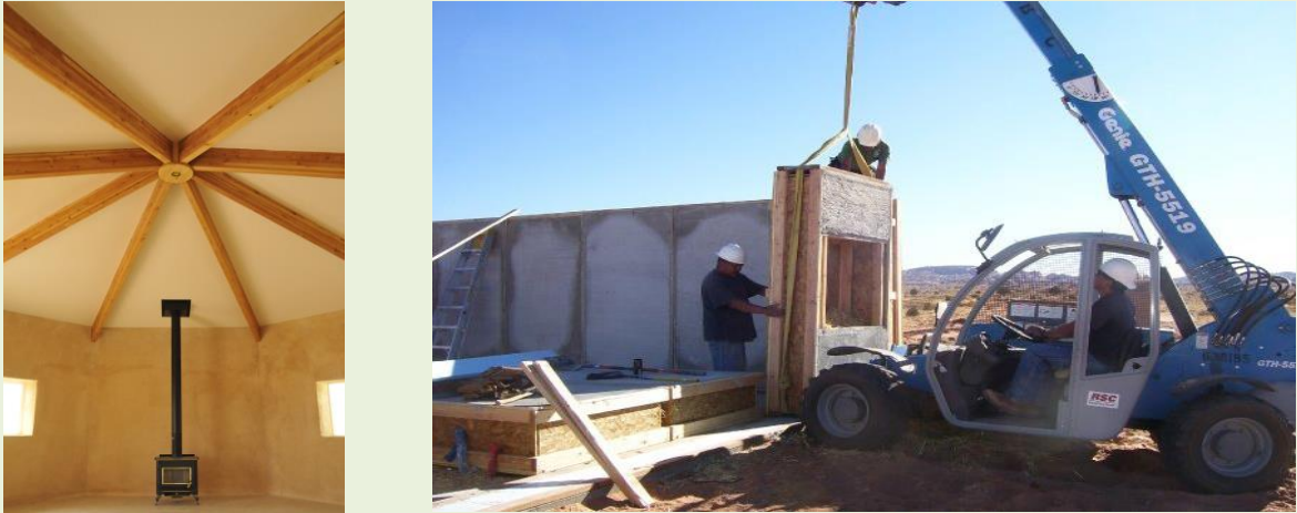
Figure 14. Left: Interior of a finished Elder Hogan home (Photo: Harry Connolly). Right: Construction of straw bale exterior walls (Photo: Nathaniel Corum). Photos used with permission from Sustainable Native Communities Collaborative.
