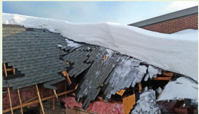
Figure 3. Partial roof collapse at an elementary school due to snow load (Building America Solution Center / U.S. Department of Education).
