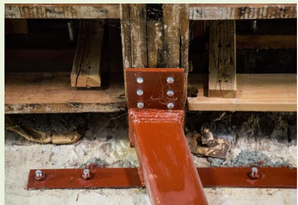
Figure 19. Photos of a secondary steel structural support inside the historic Borreo Building on Third Street in the city of Napa, California, which survived a magnitude 6.0 earthquake on August 24, 2014, with minor damage (Christopher Mardorf / FEMA).
