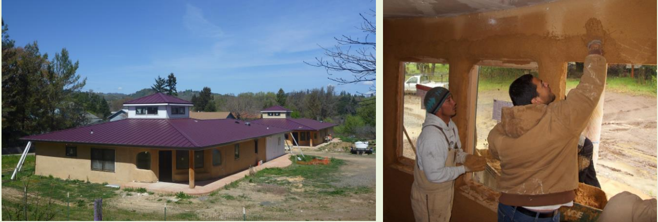
Figure 15. Left: Homes constructed for the Pinoleville Pomo Nation Homes project. Right: Applying earth plaster on an interior wall. Photos used with permission from Sustainable Native Communities Collaborative.
