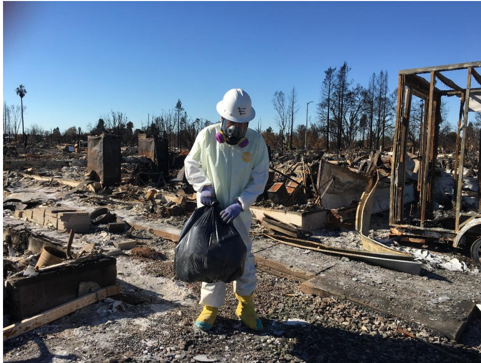
Figure 31. An EPA team member removes HHW during the Agency's response to the Northern California wildfires. Coffey Park, Santa Rosa, California.
