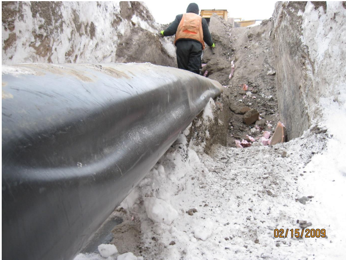
Figure 3-6. Crushed carrier line in Pt. Lay, Alaska, due to thawing permafrost (photo courtesy of UMIAQ Environmental, LLC).
