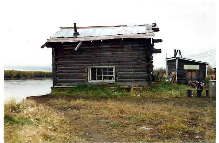
Photo 4: 2-story log home undercut by erosion, 1994.
