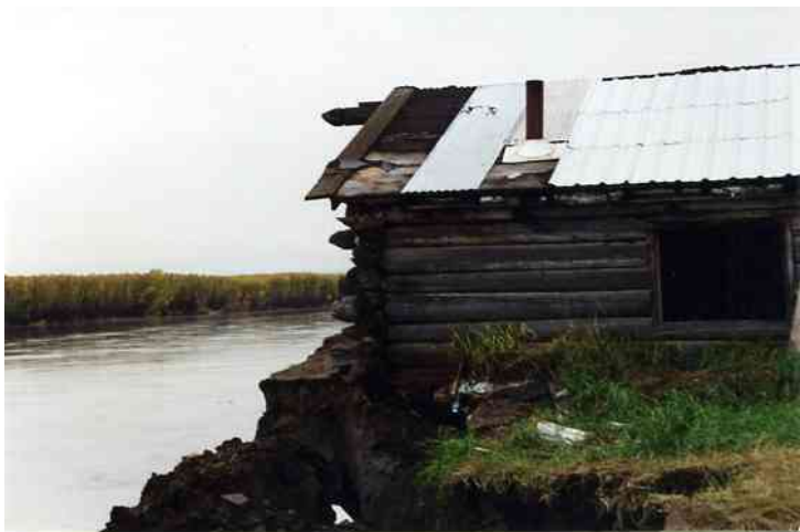
Photo 3: Log home undercut by erosion, 2004.
