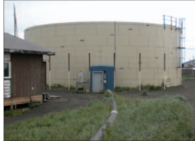
Kivalina water storage tank. Michael Brubaker, 2010.
