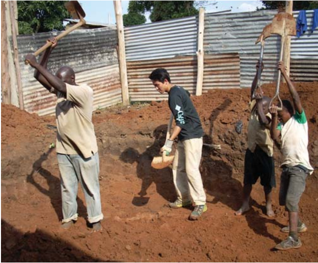
UMN student Bradley Ni, HIA teacher Joseph, and two HIA students excavate the foundation for a water tank. The ground is extremely hard, and the team needed two days to prepare sites for three tanks.
