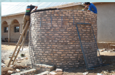
Univ Minnesota - Engineers Without Borders Rainwater Harvesting System, Uganda
