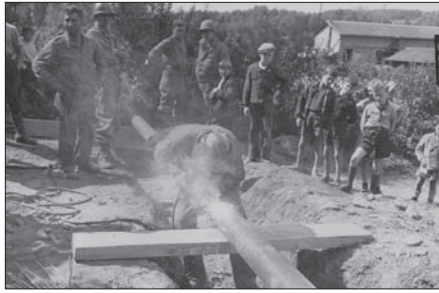
Engineers weld a gasoline pipeline into place to meet the demand for fuel by the advancing Allied forces.
