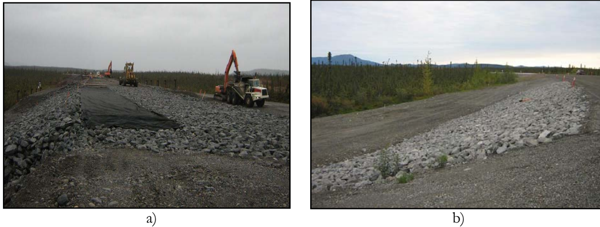
Figure 5: a) Full ACE embankment built; placing geotextile prior to base course. b) Finished uncovered ACE slopes section.
