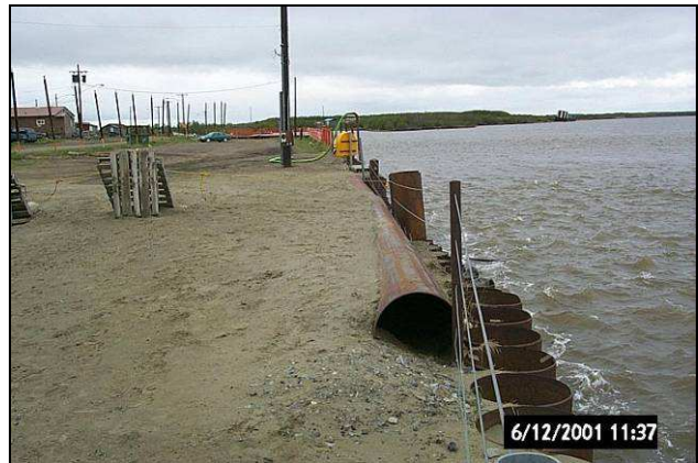
Obvious outward bowing of wall.
