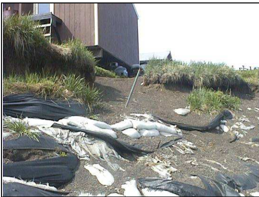
Undermined building on Kivalina
