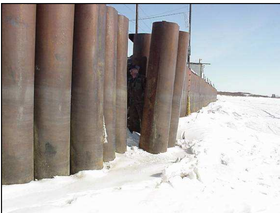
Pile wall of current concern at Bethel.
