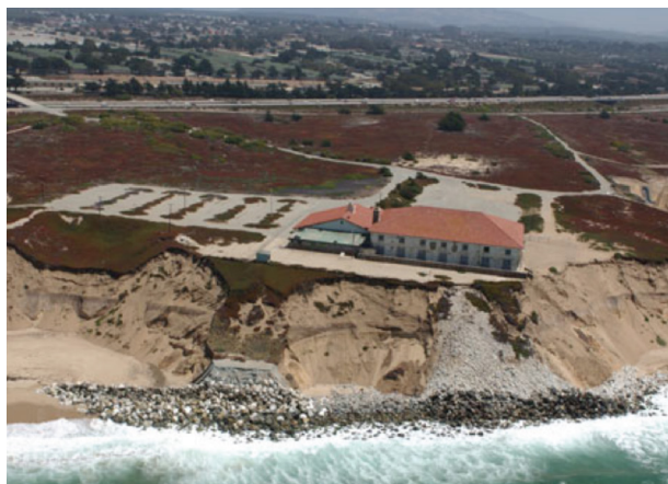
E 3. Revetment protecting Fort Ord showing placement loss, end effects, and impoundment loss. 33
