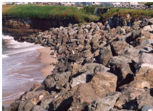
E 1. Revetment in the city of Santa Cruz showing placement loss eliminating nearly the entire beach. 26
