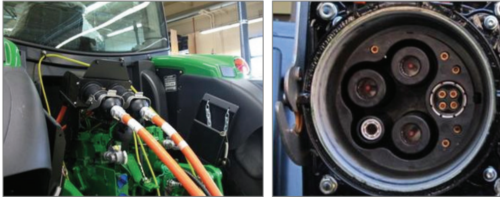
Figure 36. The high voltage electric power interface.
