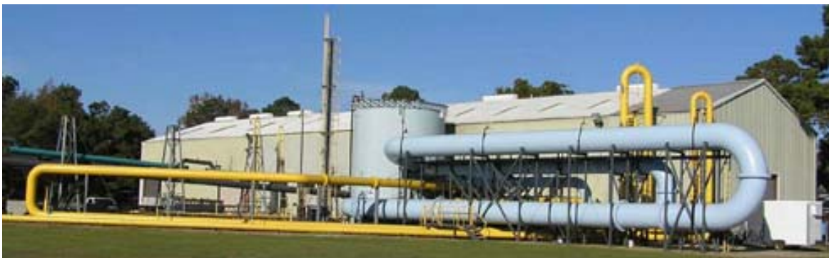
Figure 19. Exterior view of GIW Industries' centrifugal dredge pump research and testing facility in Groveton, Georgia (Courtesy of GIW Industries).
