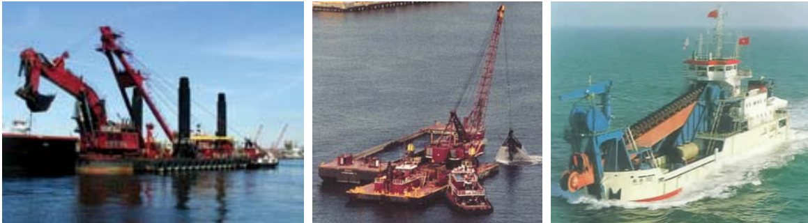
Figure 11. Backhoe dredge, New York, (left) and a clamshell dredge (center) (Courtesy of Great Lakes Dredge and Dock) a bucket ladder dredge underway (right).
