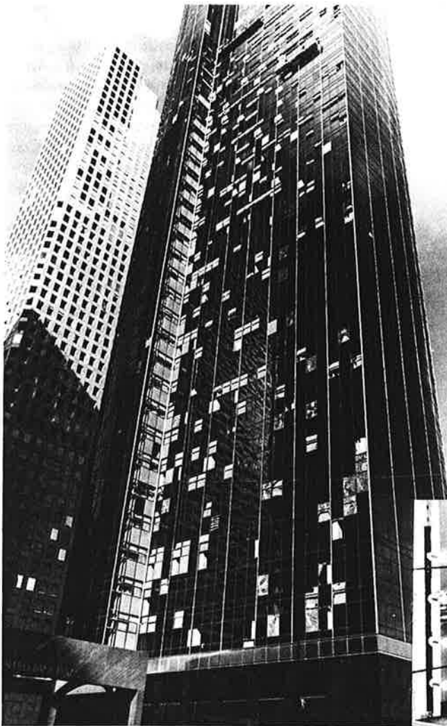
Houston buildings after Hurricane Alicia. Note window glass broken by wind pressure and windborne debris from the August 1983 hurricane.
