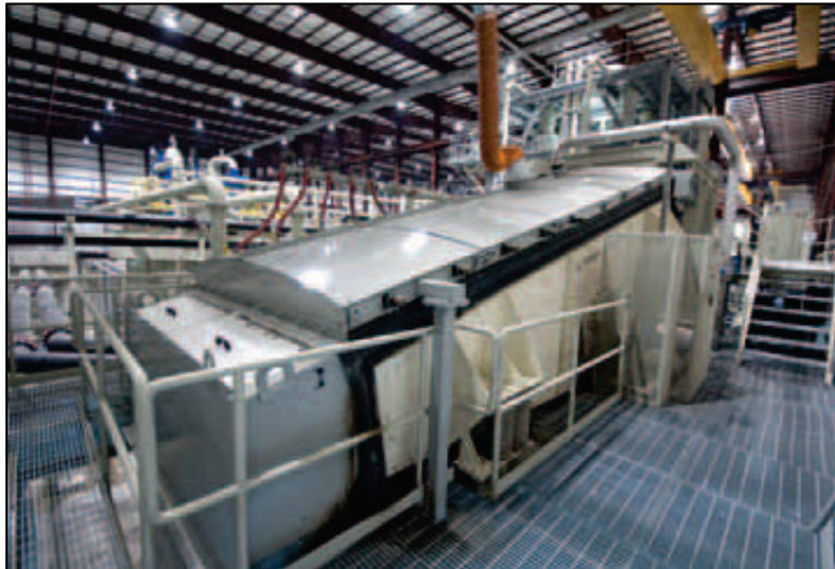
Figure D-6. Vibrating screens receive discharge from hydraulic dredges, removing oversize materials prior to pumping to the hydrocyclones.
