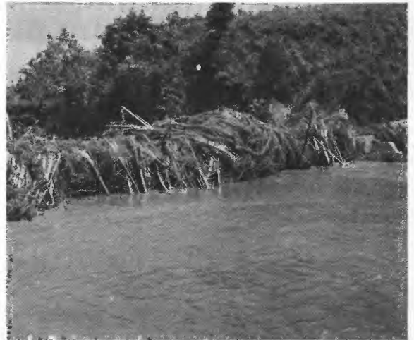
Figure 4.—Bridge opening completely clogged, mostly by bamboo.
