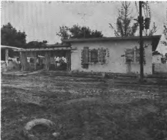
Figure 3.—After the recession of the floodwaters at the northwest edge of Humacao. Note the man pointing to the high-water mark above his head.
