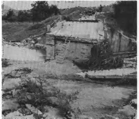
Figure 9.—Bridge on Rio Limones near Limones. Wingwall from left side was found intact about 50 feet downstream; the remains of the wingwall from the right side can be seen in the foreground.
