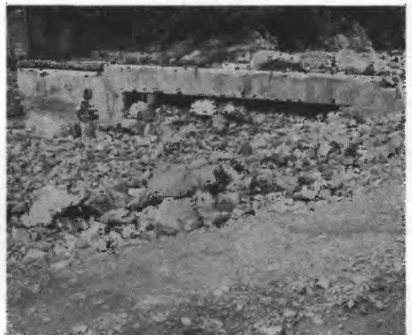
Figure 5.—View from downstream side of bridge on Rio Turabo near La Plaza. Note the rock-filled channel above the bridge.
