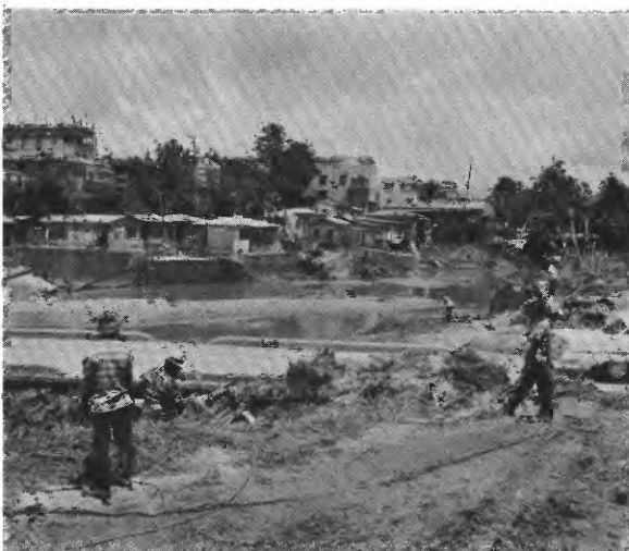
Figure 7.—View showing damage to floodwall along left bank at Rio Valenciano in Juncos.
