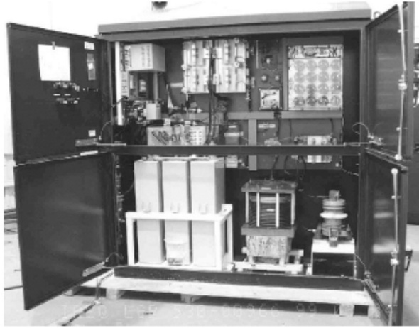
Figure 27: Neutral current blocking device (NCBD) installed in the neutral of a three-phase transformer as a year-long test by Hydro Quebec [7].
