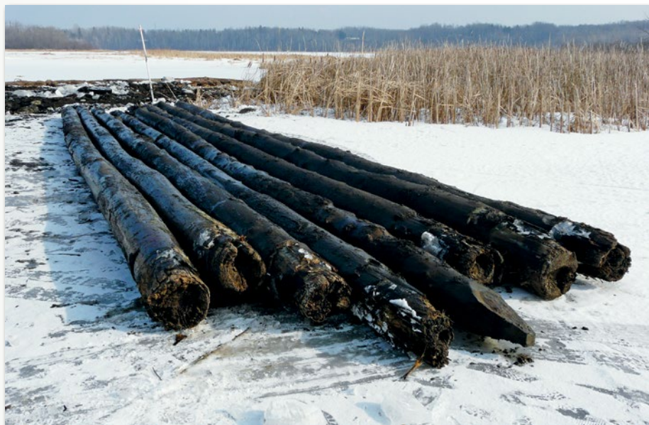
Here are just a few of the 460 pilings that were pulled from the bottom of the polluted Radio Tower Bay.
