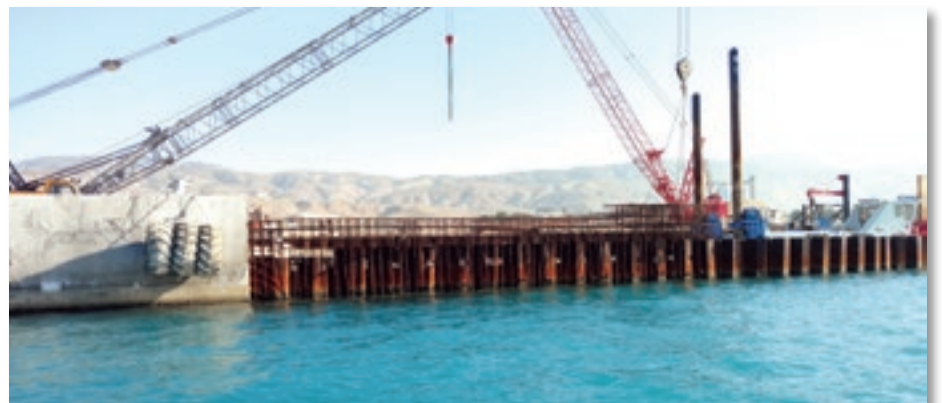
Part of the quay wall remains unfinished in 2018.
