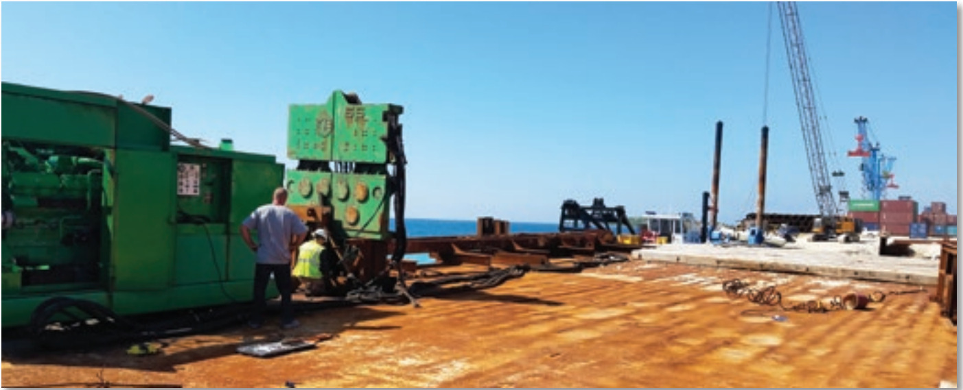
Part of the battle at the start of emergency repairs was getting equipment fixed and working.
