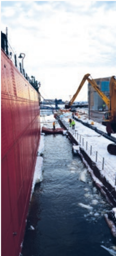
The Irvin was moved last winter for the first time since 1986 for repairs to be made on failing seawalls.
