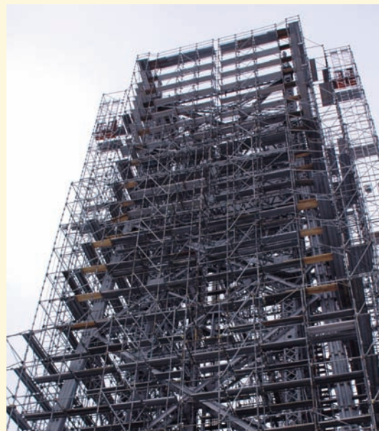
Building a lacy network of scaffolding around the Aerial Lift Bridge's south tower is the first step toward painting it.
