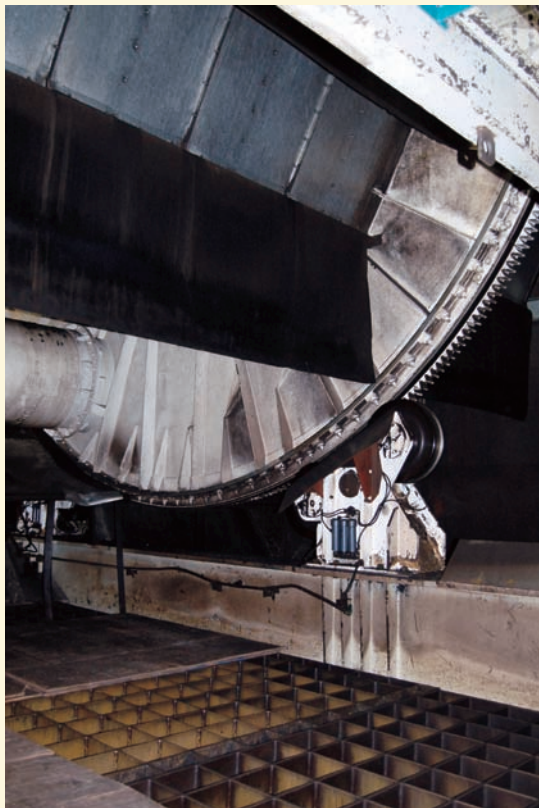
The rotary car dumper at Midwest Energy was due for some major work during this layup season.
