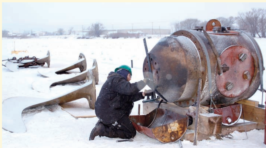
Work on the H. Lee White , in drydock at Fraser Shipyards, includes dismantling and inspecting the propeller hub and blades.
