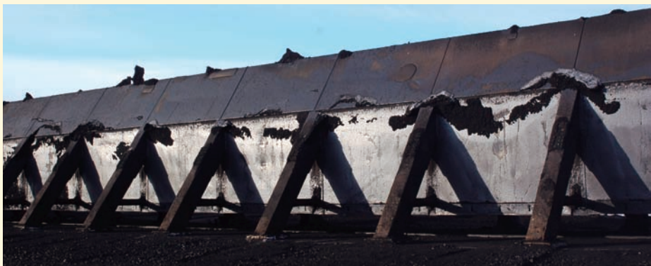
This coal feeder system and the ground around it at Midwest Energy spend most of their lives under mountains of coal. They are exposed briefly during the shipping lull for inspection and maintenance.
